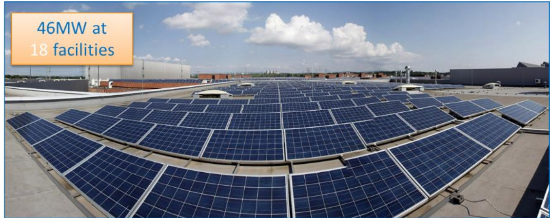
Opel Rüsselsheim facility in Germany, 8MW rooftop array
