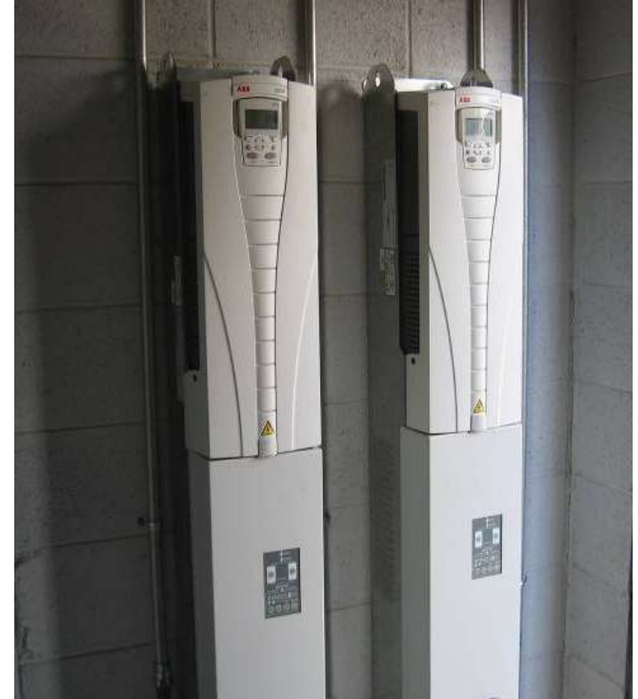
VFDs for HVAC fans and pumps
